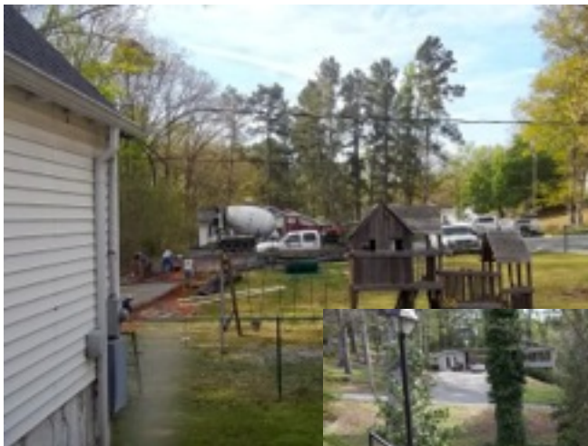
(Left) Construc- tion of driveway from parking lot to parish hall en- trance.
